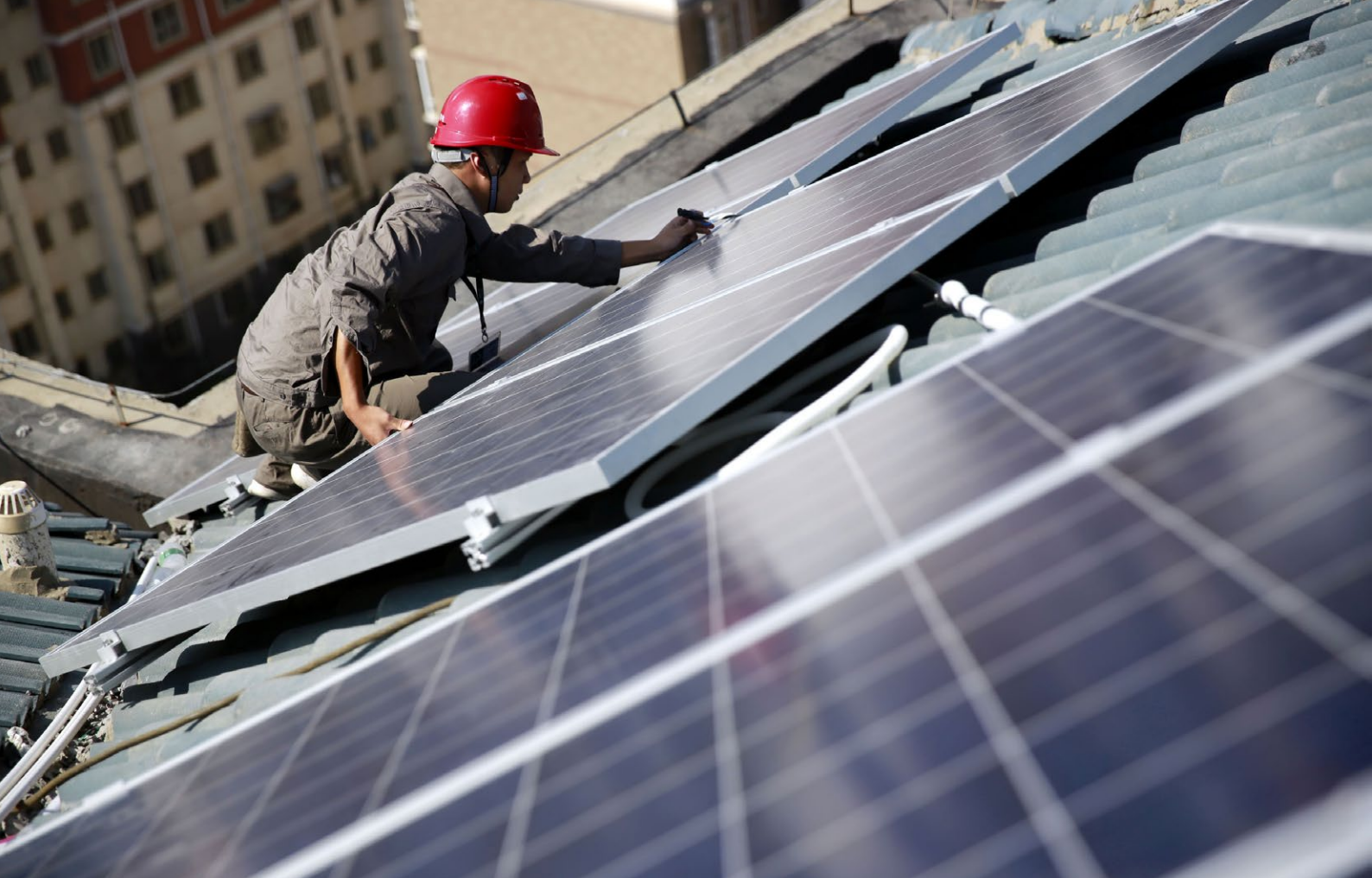
Solar panels on the rooftop of a housing development in Jiujiang. Credit: humphery / Shutterstock.
